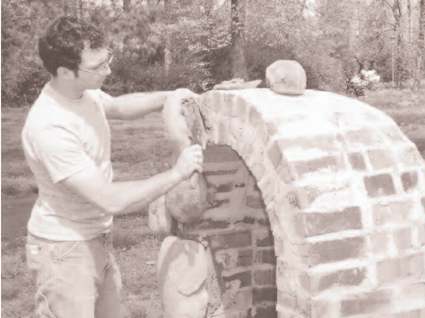
Sam Vitale ('05) works on the construction of the new Grotto of Our Lady, the Holy Mother of God.
